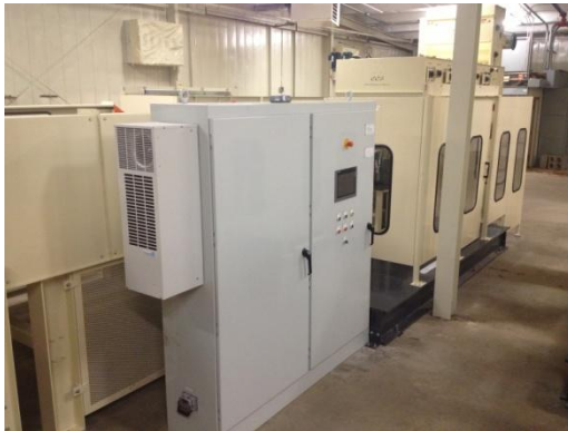
AIR CONDITIONED CARD PANEL
