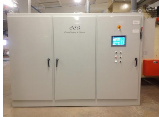
BLEND LINE CONTROL PANEL
