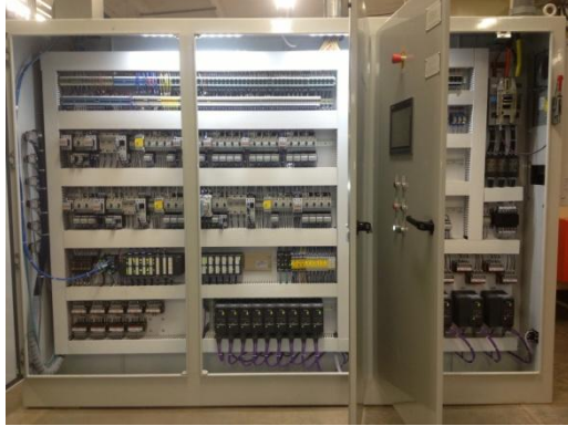
BLEND LINE CONTROL PANEL
